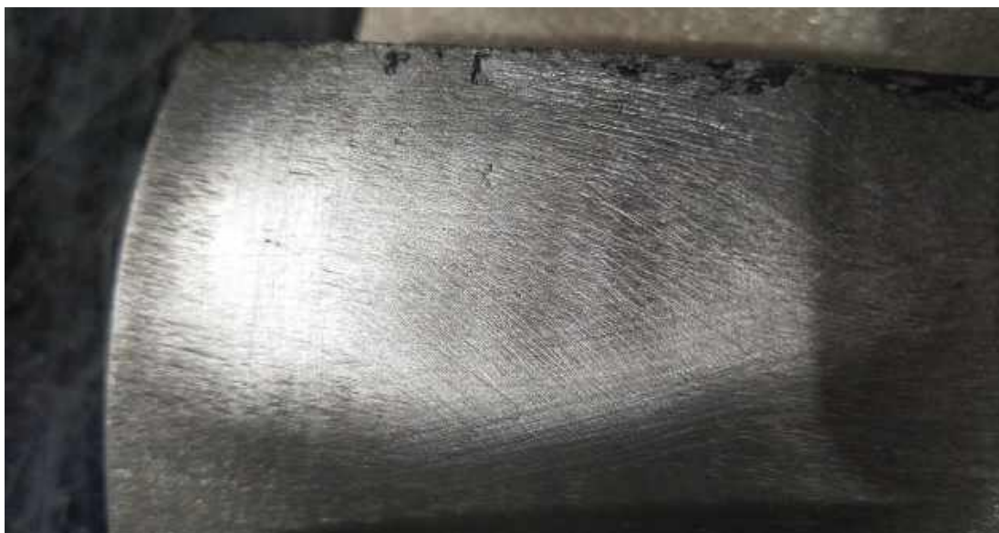
Figure 5.11 – The blade where the defects were found; the detected flaws are almost invisible to the naked eye
